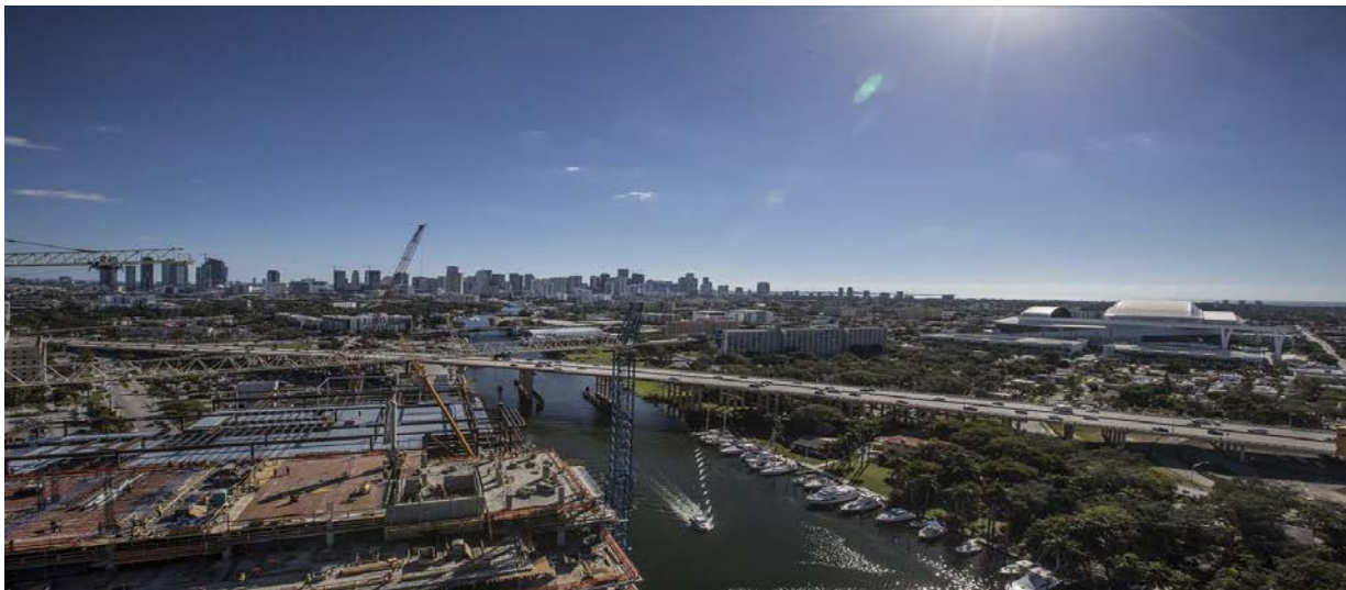
A boat heads west on the Miami River past the River Landing construction site on Monday January 7, 2019.
